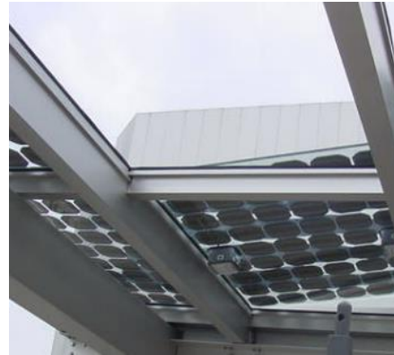
PV Installation with Al structure
